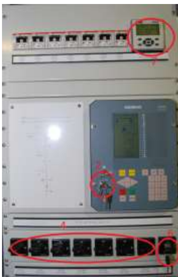
Figure 11: Bay Control Point in SCS control
