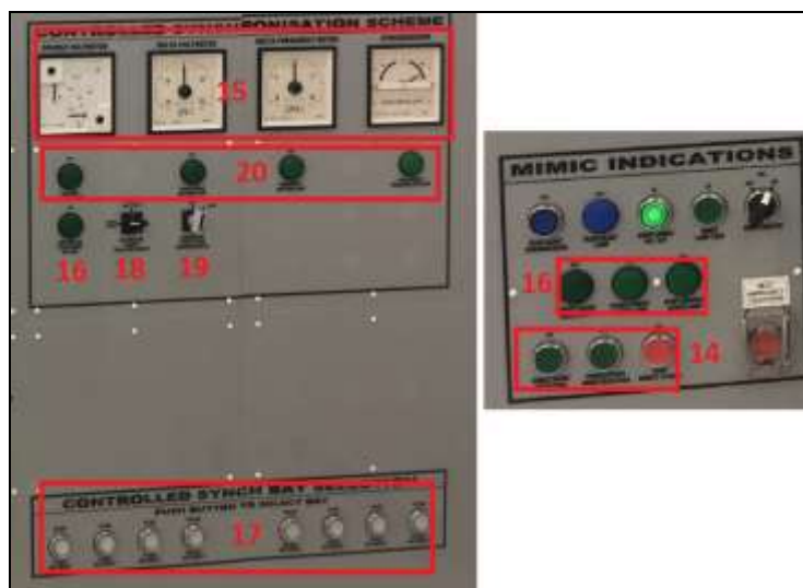
Figure 12: Check Synchronising Switches and Indications
