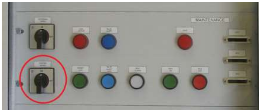
Figure 3: Master Remote Control On/Off installed on SLC
