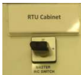
Figure 2: Master Remote Control On/Off installed on RTU
