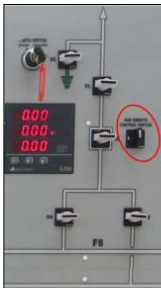
Figure 9: Bay Sub Remote Control On/Off switch (RTU substation)
